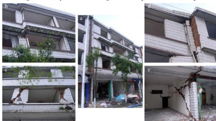
Figure 1. Damaged 4-storey URM building due to in-plane and out-of plane actions [3]
