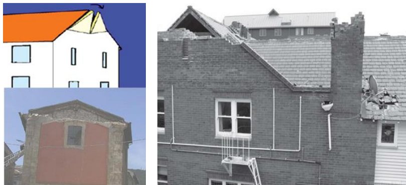
Figure 4. Overturning of gable wall [4] and chimney [5] due to lack of anchorage
