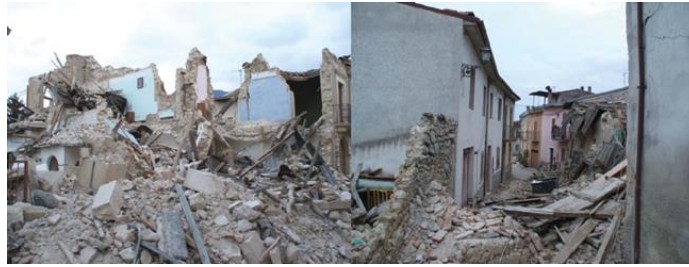
Figure 2. Collapse due to poor and disaggregated masonry [4]
