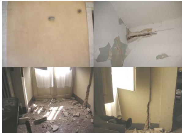
Figure 3. Mixed collapse mechanisms: out-of-plane and in-plane damage [4]
