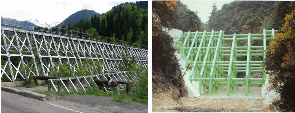
Figure 9. A flood catcher made of steel elements
